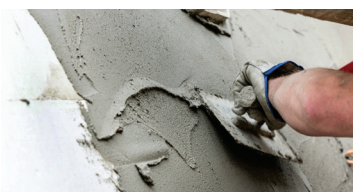
DryMix Building Materials Processing
